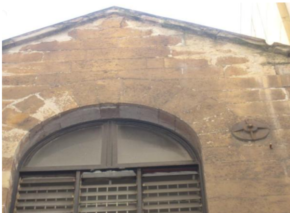
DETAIL OF THE GABLE END SHWOING DELAMINATED (SPALLING) STONE BENEATH THE PARAPET CAPPING
