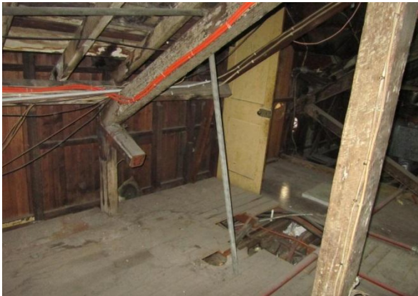
DETAIL OF ONE OF THE MISSING MEMBERS
