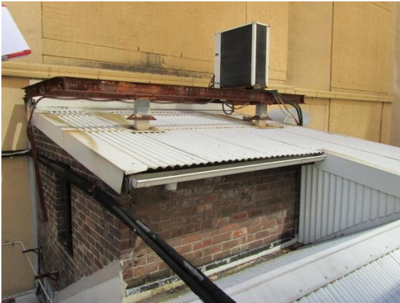
LIFT MOTOR ROOM
