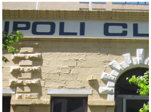
CRACKING TO THE PARAPET
